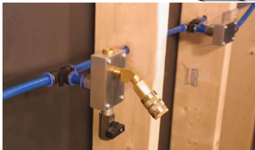
Hidden Mount air line is inside the wall
